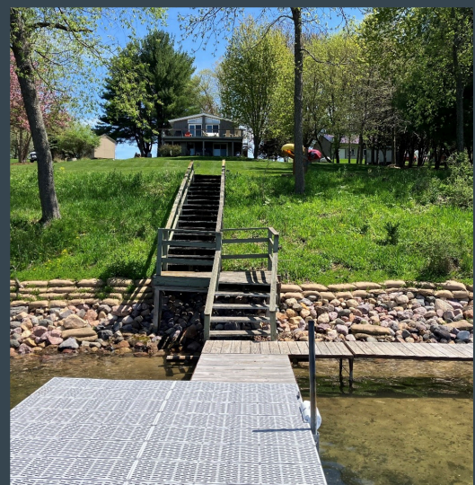
Lake Redstone Shoreline Stabilization Project using rock riprap, geotextile bags, and native plants
