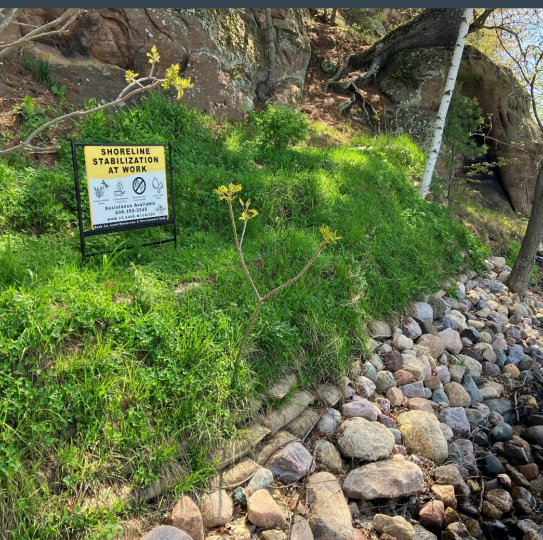
Dutch Hollow Shoreline Stabilization Project using vegetated rock riprap, geotextile bags, and native plants
